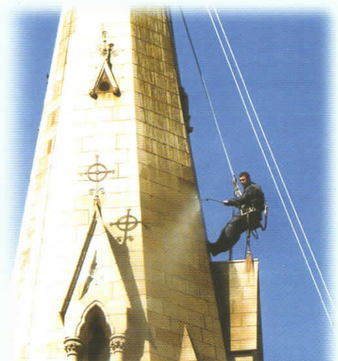
Conservation Cleaning in Progress, St Patricks, Killygordon by Brian Rainey Jr. Architect, M.H. Associates
